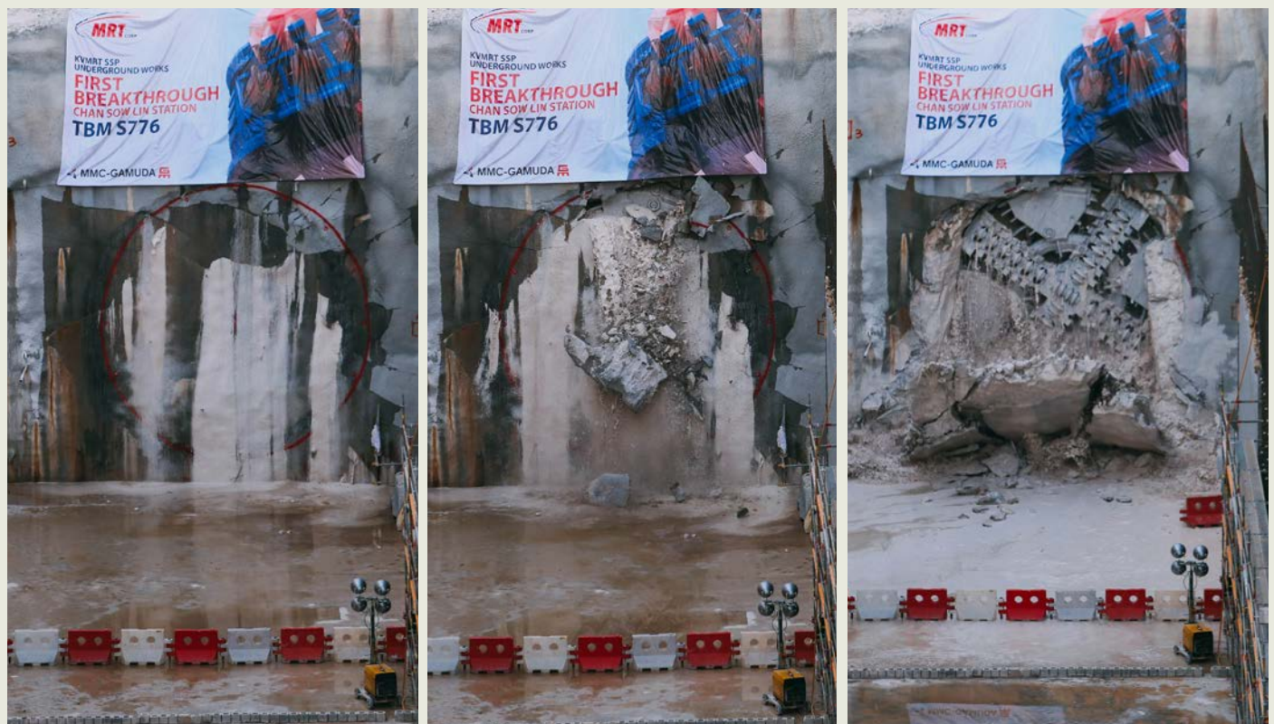
■ BREAKTHROUGH: Sequence of photos showing the tunnel boring machine breaking out from the ground after excavating a stretch of tunnel.
