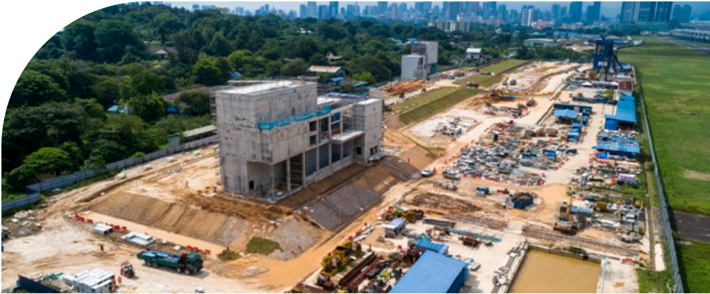
Turfing and external plastering works for Bandar Malaysia Selatan MRT Station entrance in progress.
