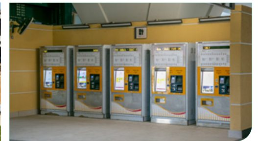
Installation of ticket vending machine is completed at the Serdang Jaya MRT Station.
