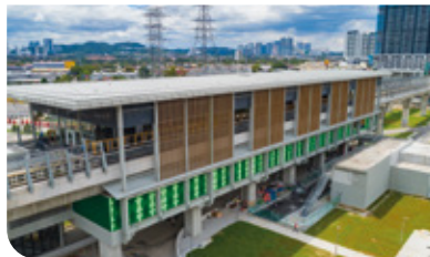
Overall view of the Ampong Park MRT Station showing the architectural works in progress.
