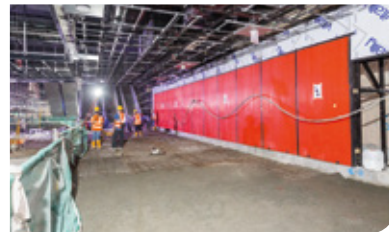
View inside the Ampong Park MRT Station showing the architectural works in progress at the lower concourse Front of House.
