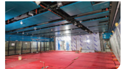
Installation of Automatic Fare Collection system gate at the concourse level of the Titiwangsa MRT Station.
