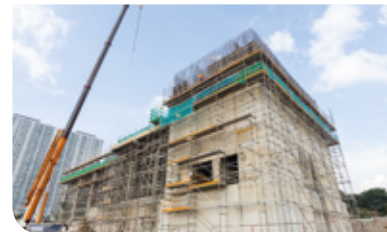
Construction of the entrance and ventilation building of the Bandar Malaysia Selatan MRT Station.
