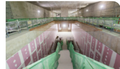
An inside view of the Bandar Malaysia Utara MRT Station showing readiness of the Front of House and completion of drywall partition at platform level.
