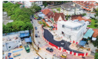
Aerial view of the Escape Shaft 2 showing the road reinstatement works and BOMBA parking construction in progress.
