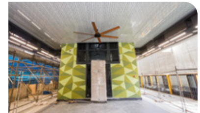
View inside the Jalan Ipoh MRT Station showing the mural painting works on lift.
