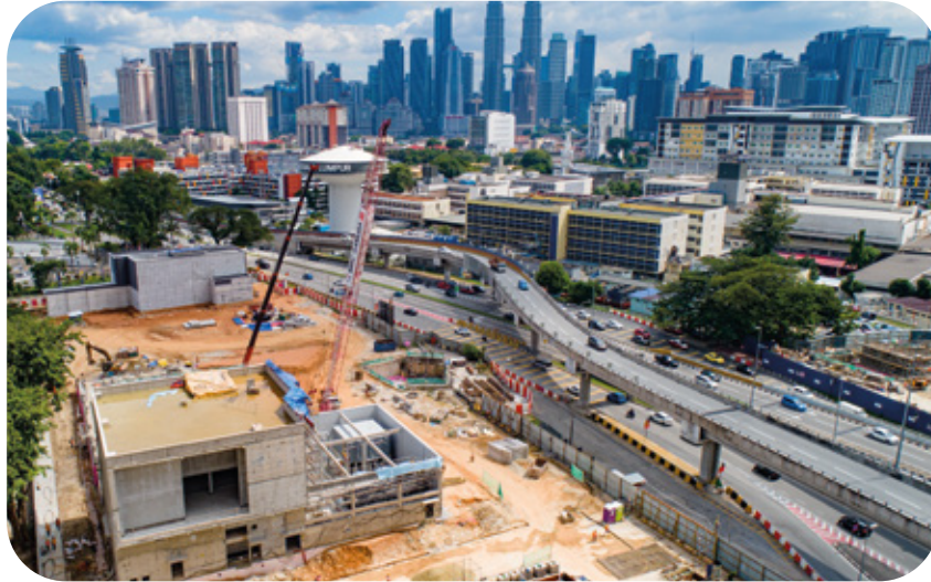
Aerial view of the Hospital Kuala Lumpur MRT Station showing the ongoing architecture finishes at the Entrance B and C while building reinforcement works in progress at the Entrance A.
