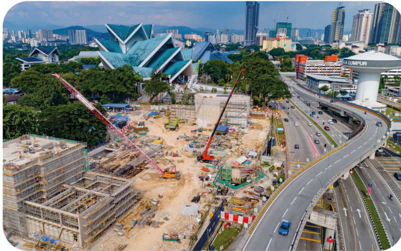
Aerial view of the Hospital Kuala Lumpur MRT Station showing the completion of reinforced structure at the Entrance B and C with ongoing reinforced works at Adit and Entrance A.
