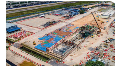
Aerial view of the Bandar Malaysia Utara MRT Station showing the structural works in progress for Vent A and Entrance A.
