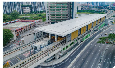
Aerial view of the Sri Delima MRT Station showing the defect rectification works in progress.
