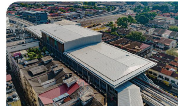
Aerial view of the Kentonmen MRT Station showing the plastering works and electrical and mechanical ducting works in progress.
