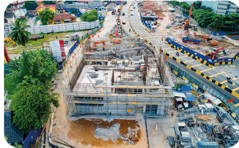
View of the Conlay MRT Station showing the cladding works at the concourse level.
