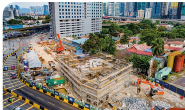
Aerial view of the Raja Uda MRT Station showing the construction of Ventilation Building B in progress.
