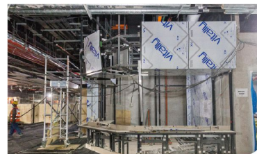
View of the Persiaran KLCC MRT Station showing the installation works for Aluminium Composite Panel for Customer Service Room.
