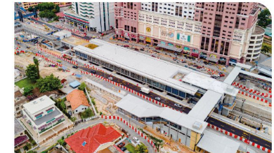
Aerial view of the Jalan Ipoh MRT Station showing the tiling works in progress at the edge of the platform.
