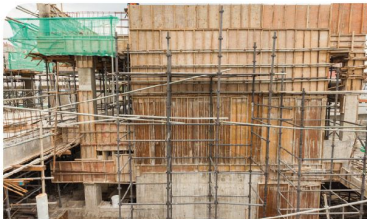
View of the Multi-Storey Park and Ride of Metro Prima MRT Station showing the lift pit wall in progress.
