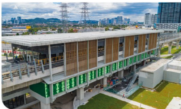
Aerial view of the Jinjang MRT Station showing the pier repair for finishes in progress.
