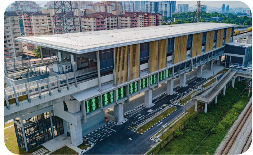
Aerial view of the Kampung Batu MRT Station showing the defect rectification works in progress.
