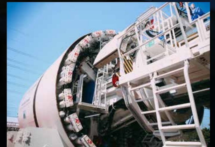
TUNNEL EXCAVATION: The pressurised excavation chamber of the Variable Density Tunnel Boring Machine that removes the excavated materials.
