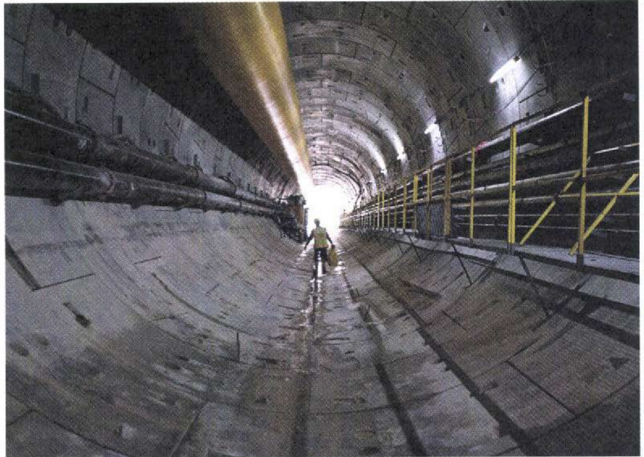
The RM15.47 bil underground work package was awarded to MMC Gamuda KVMRT
