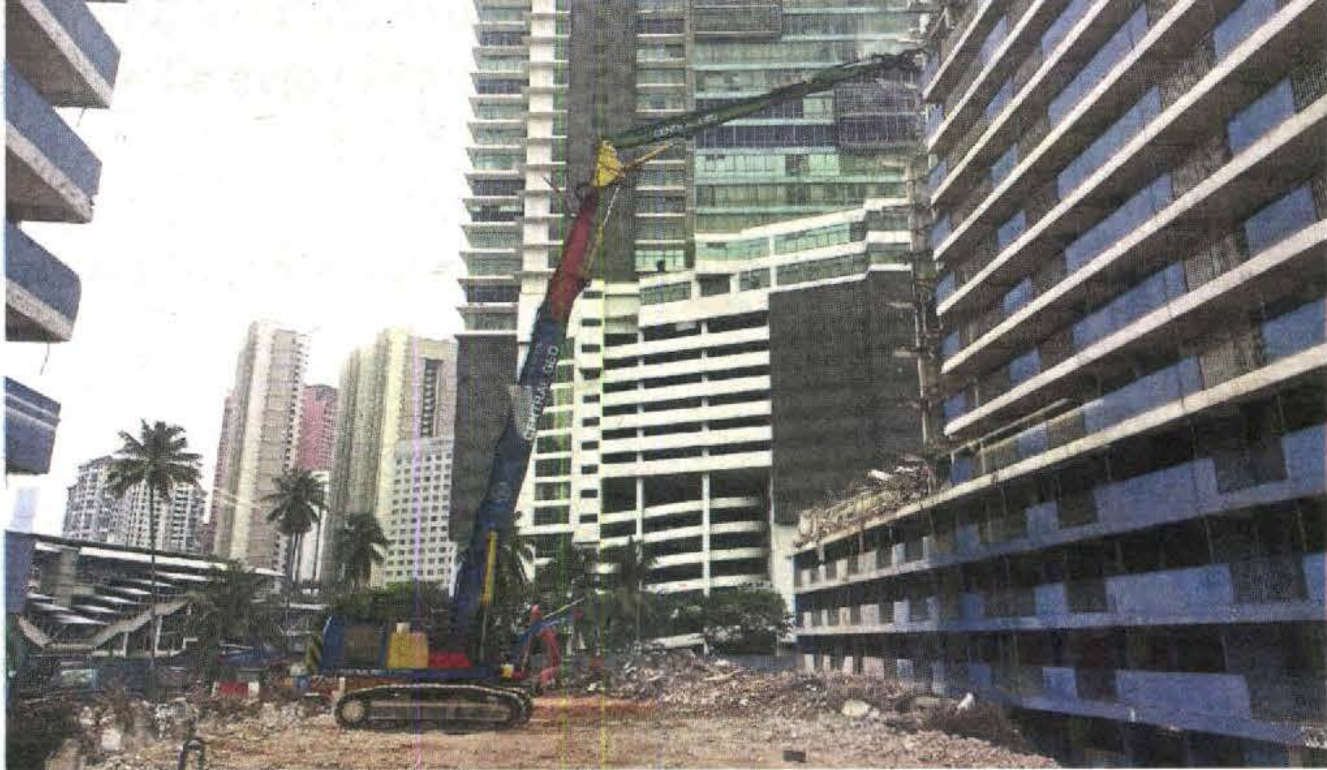
An excavator can be seen at the site of the Sentul police quarters in Jalan Sentul Manis, Kuala Lumpur, that will be demolished soon to make way for the MRT SSP Line.
