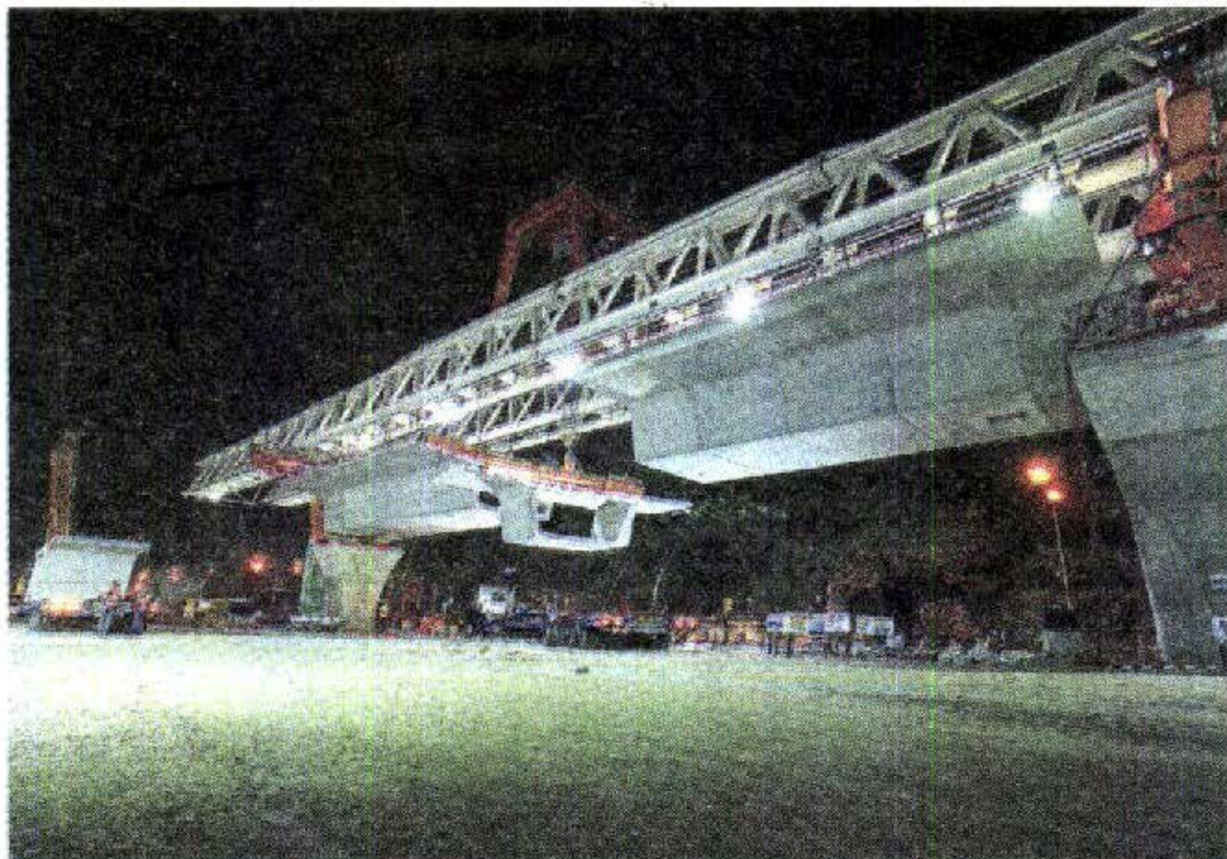
Segmented box girders being lifted by the launching gantry. Manulife Semantan MRT Station is approximately 5 minutes' walk away from Menara Manulife
