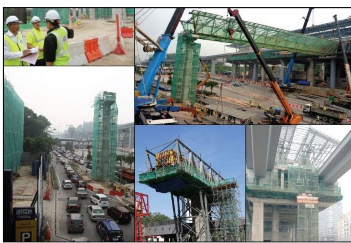
Government had given the final approval for the MRT Sungai Buloh-Serdang-Putrajaya Line (SSP Line) railway scheme
