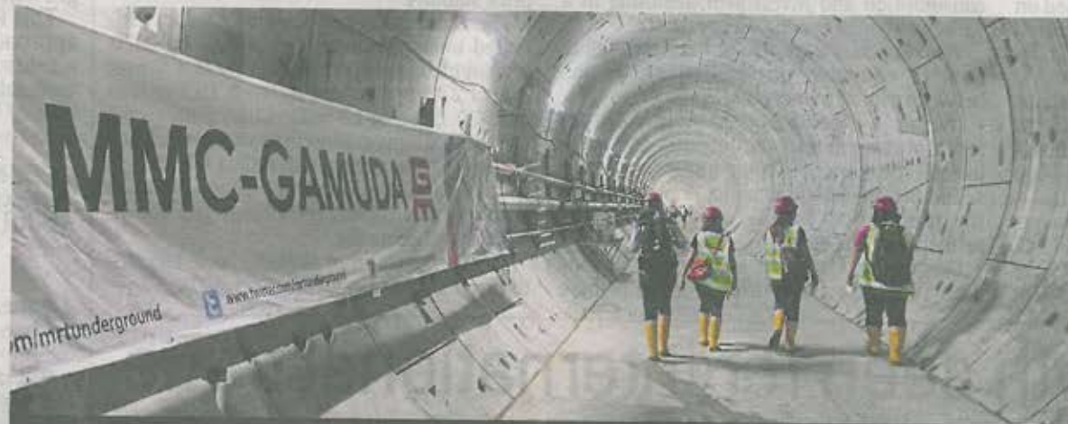
MRT Line 2 has only awarded MMC Corp Bhd and Gamuda Bhd as the project delivery partner of the second rail construction based on its track record for the MRT Line 1.
