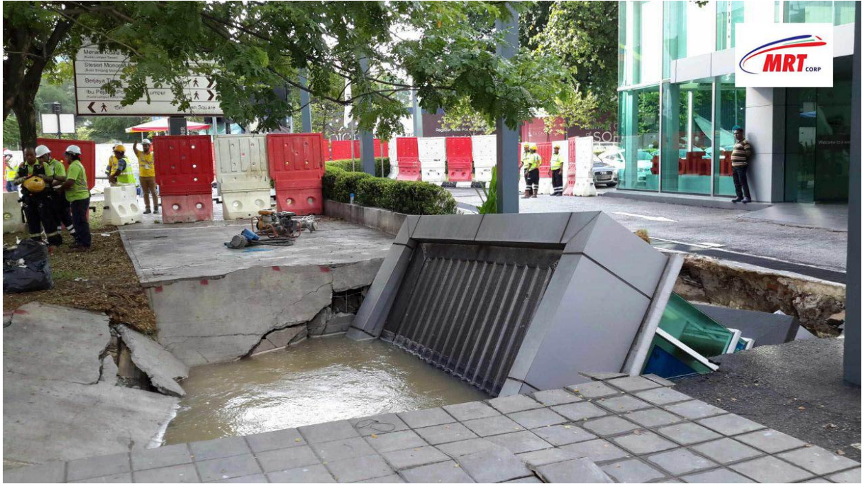
The guardhouse of a nearby car dealer in the sinkhole which had been filled with water from the burst pipe.
