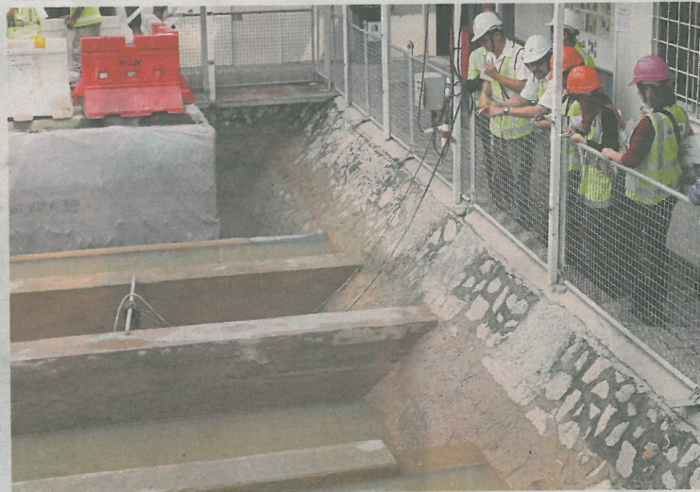
The drainage system in MRT Pasar Seni project site carries de-silted water to Sungai Klang. Pic by Farizul Hafiz Awang
