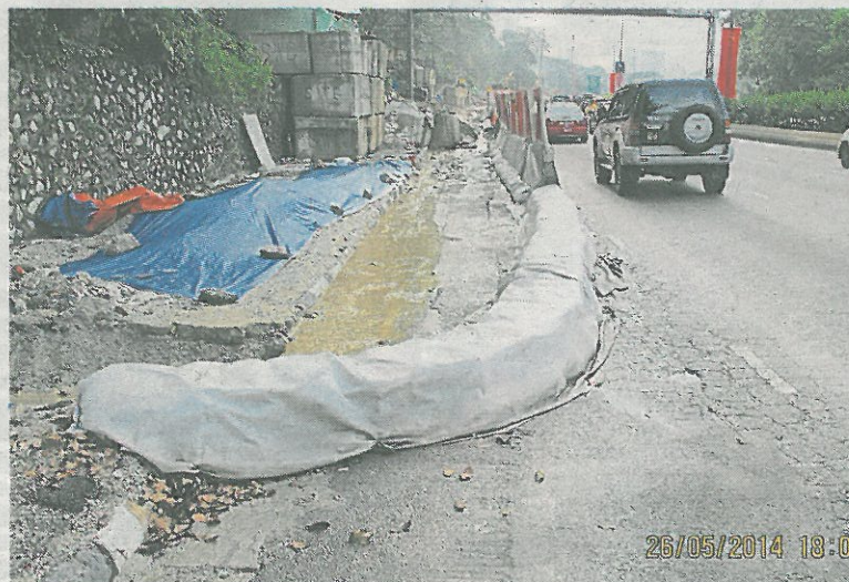
Preventive measures: Sandbags arranged along Jalan Duta, at a MRT worksite, to prevent muddy water from flowing to the main road during a heavy downpour.
