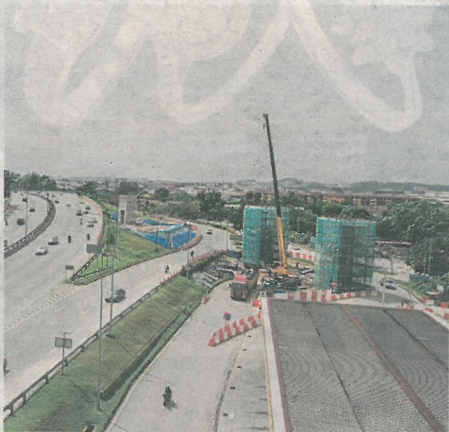
The special span across the Cheras-Kajang (Grand Saga) Highway is one of 21 special spans to be built for the Sungai Buloh-Kajang MRT line.
