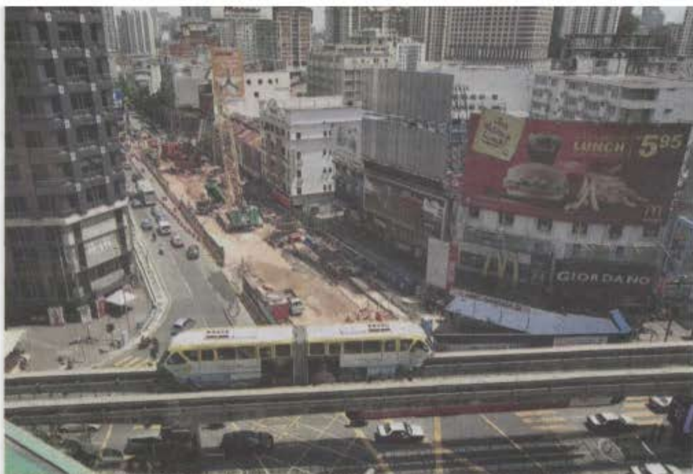
HIDDEN WORKS: Tunnelling and boring are being done underneath the MMC-Gamuda KVMRT (T) Sdn Bhd's worksite in Jalan Bukit Bintang
