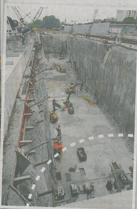
Aerial view: View of the 30m-deep Cochrane shaft. The dotted lines indicate the area where the works are being carried out.
