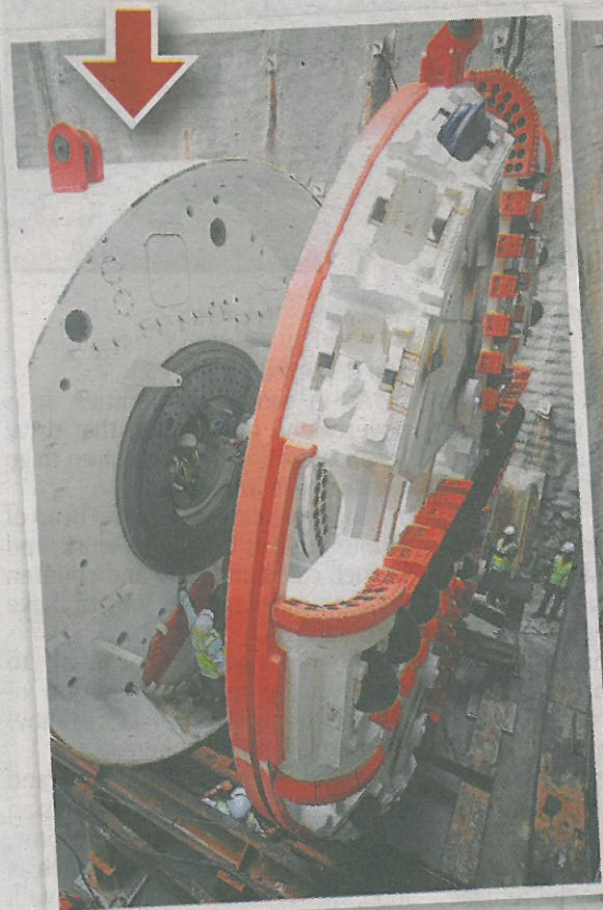
Working on it: There is still a lot of horizontal movement required to move the cutterhead closer to the first segment of the TBM.
