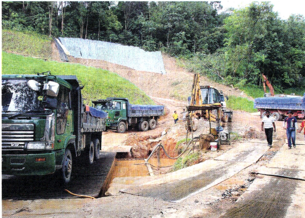
Muddy times: Residents are concerned over potential landslips at the Sanctuary Ridge project during the rainy season.
