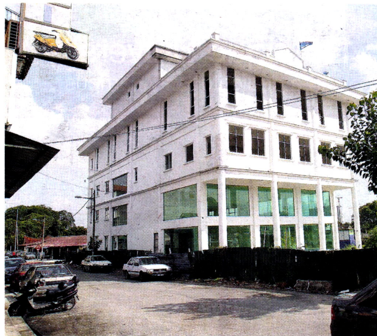
Almost ready: The 90% completed Hulu Langat MCA division building at Jalan Hishamuddin in Kajang that will be demolished.
