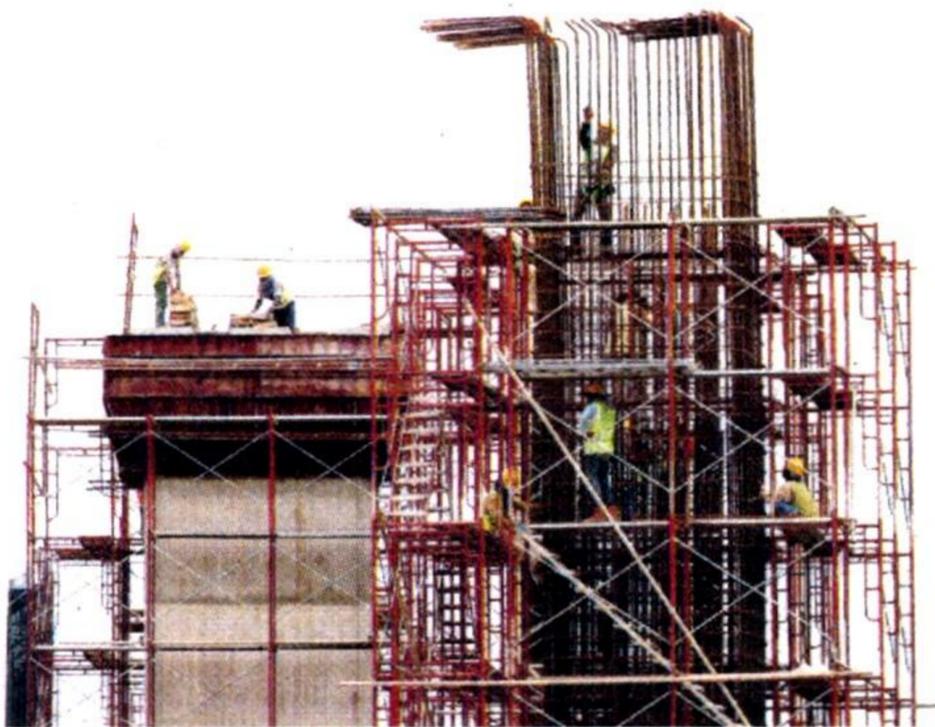
Workers prepare scaffoldings to pour concrete into a giant column for the 150-km Mass Rapid Transit system in Kuala Lumpur. — AP
