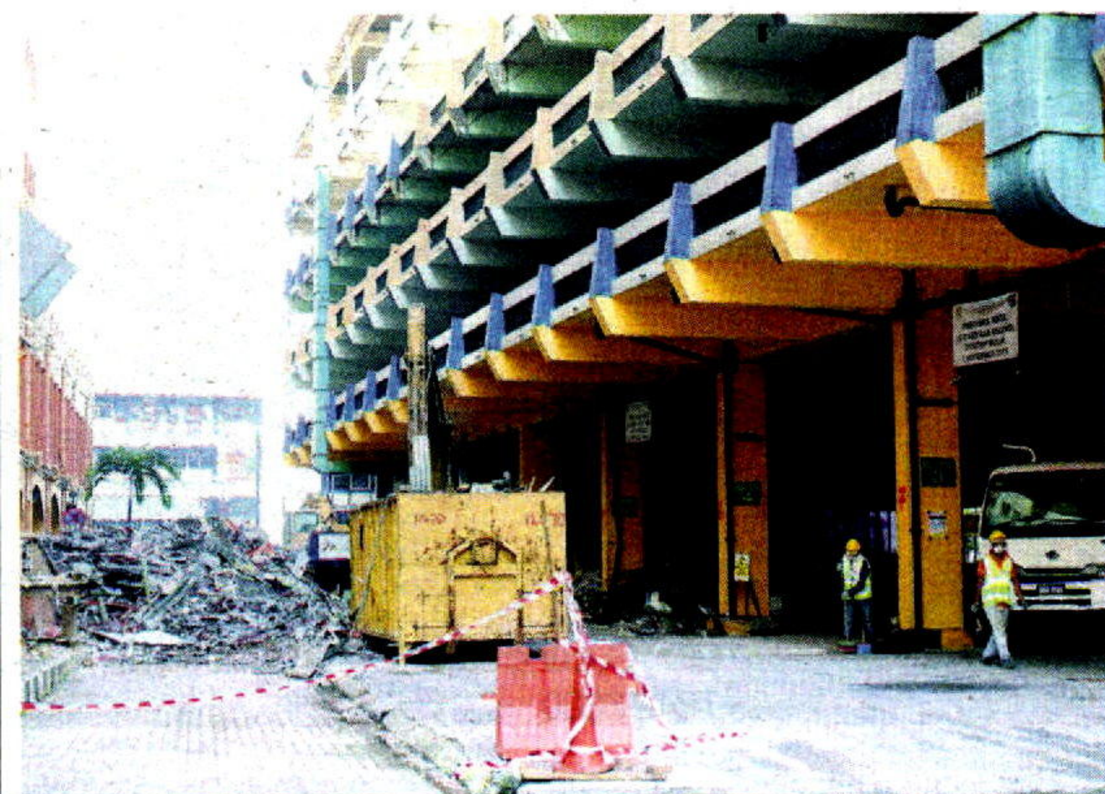
All to come down: The preparation work for the demolition of Klang Bus Stand had already begun.
