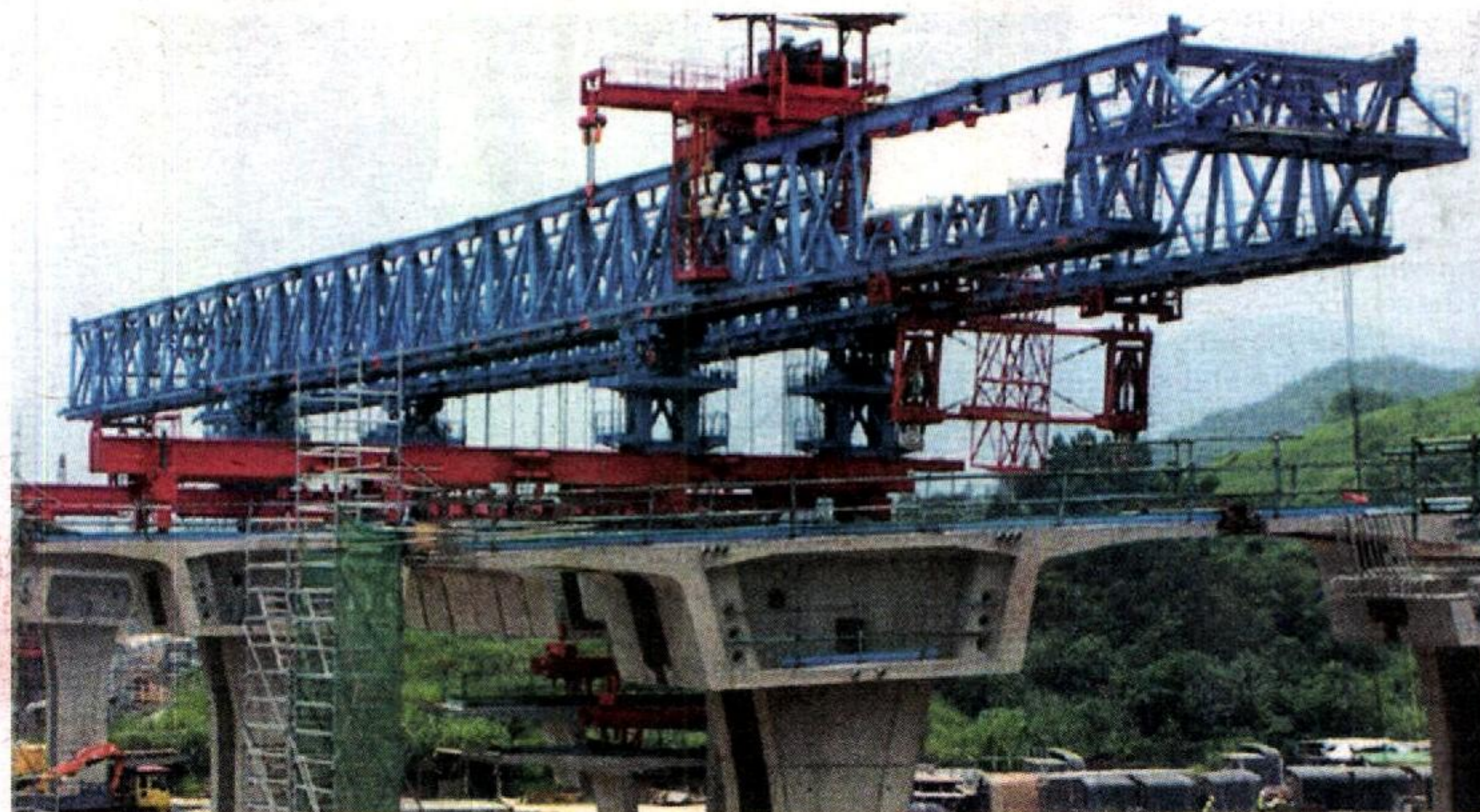
→ Turn to Page 2 The MRT gantry of Package V6 precast segments will be soon be put in place.
