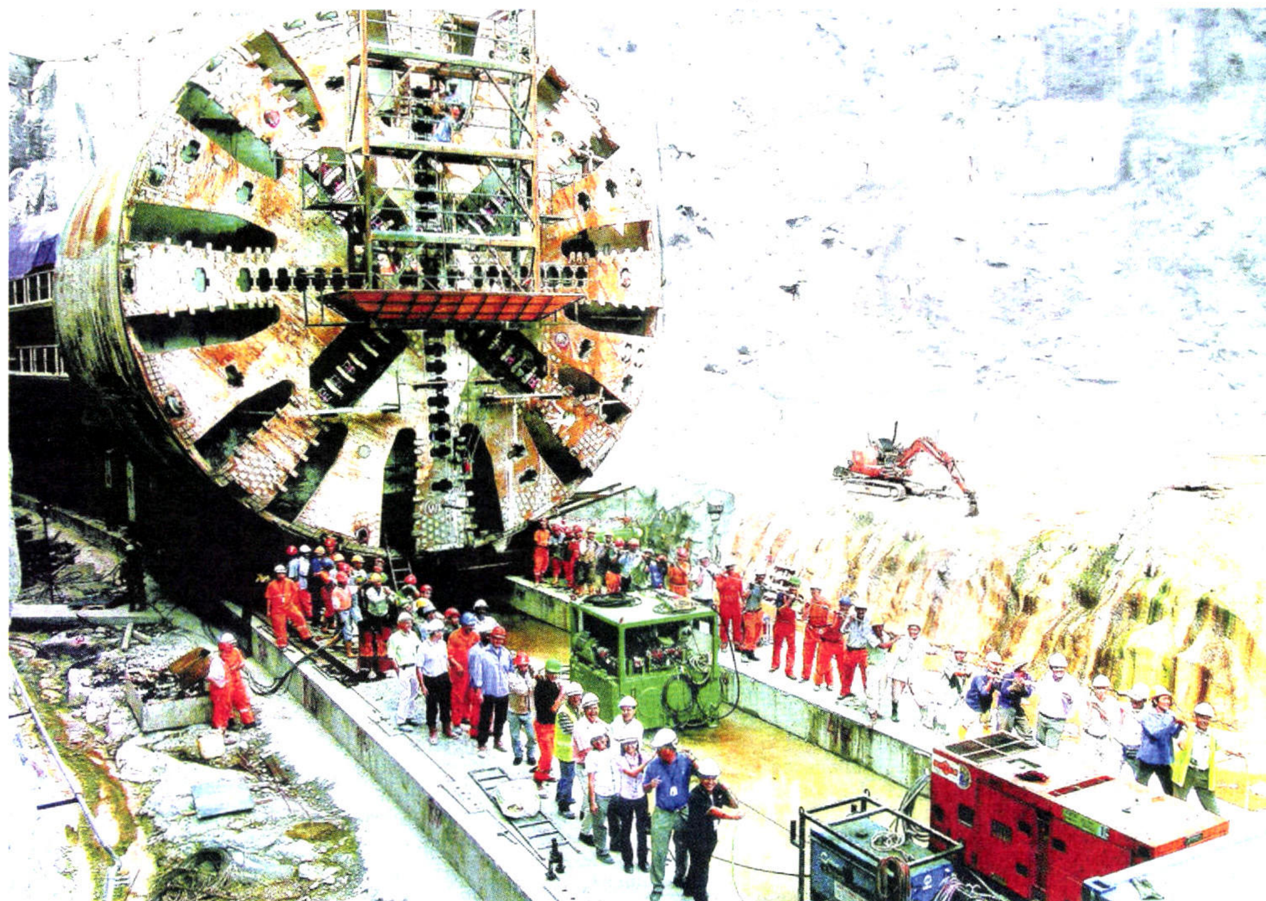
Maybank Kim Eng estimates a multiplier impact of 6.8 times on the domestic economy should a local player snag the tunnelling works.
